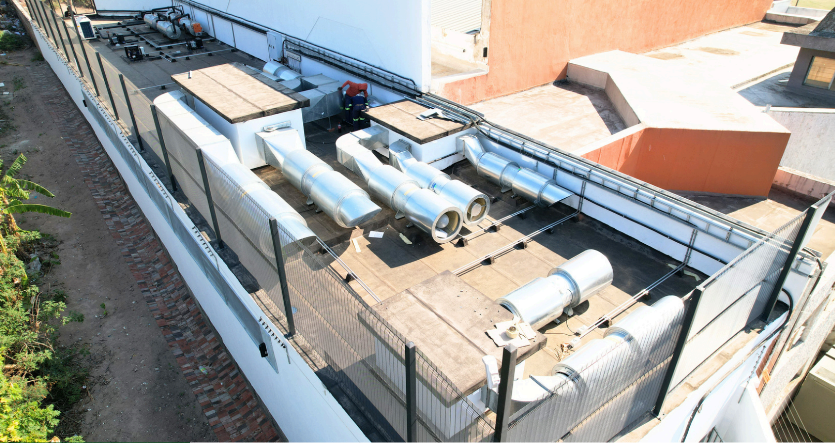
Roof Level installed with Ventilators, Makeup Air ducts, Compressors and Electrical supply to the Compressors
